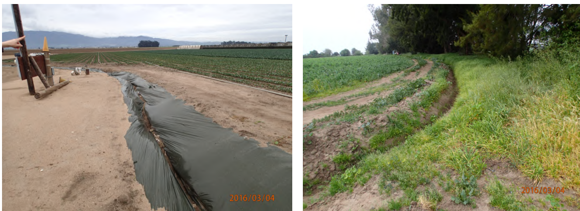
Figure 2. On the left, an example of the use of plastic alongside the road for erosion control. On the right, an example of gully erosion alongside the road.
