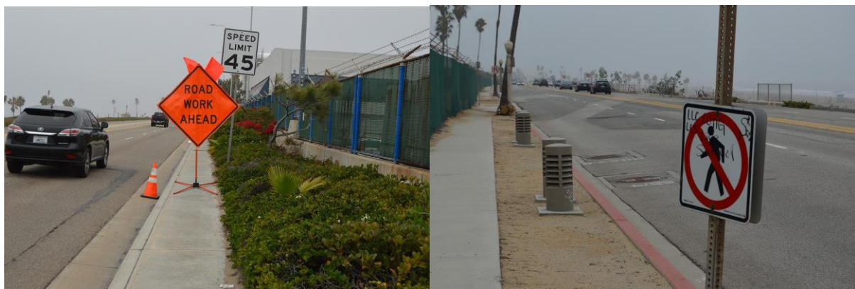
Left, fig. 5. Road work ahead sign completely blocks the miniscule sidewalk next to Vista Del Mar from: Stone, Billy. 4 th November 2021, Author’s personal collection
