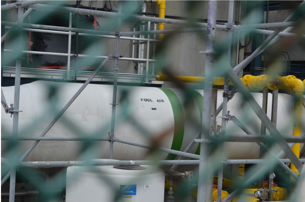
fig. 21. A large pipe funnels “foul air” near the entrance to Hyperion plant from: Stone, Billy. 4 th November 2021, Author’s personal collection
