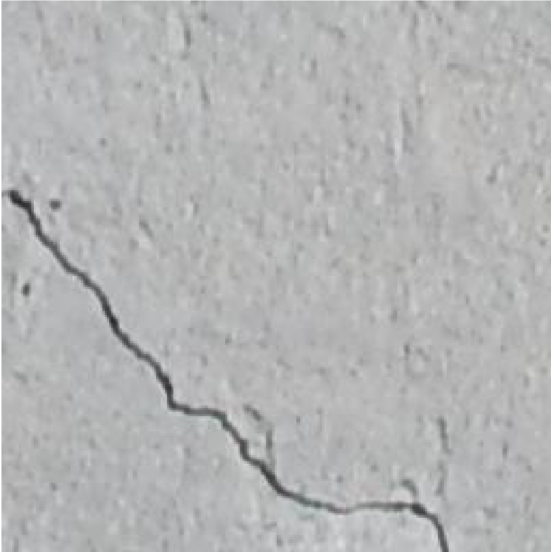
Figure 7.18: Image 7002-28 of a Bridge Deck Crack
