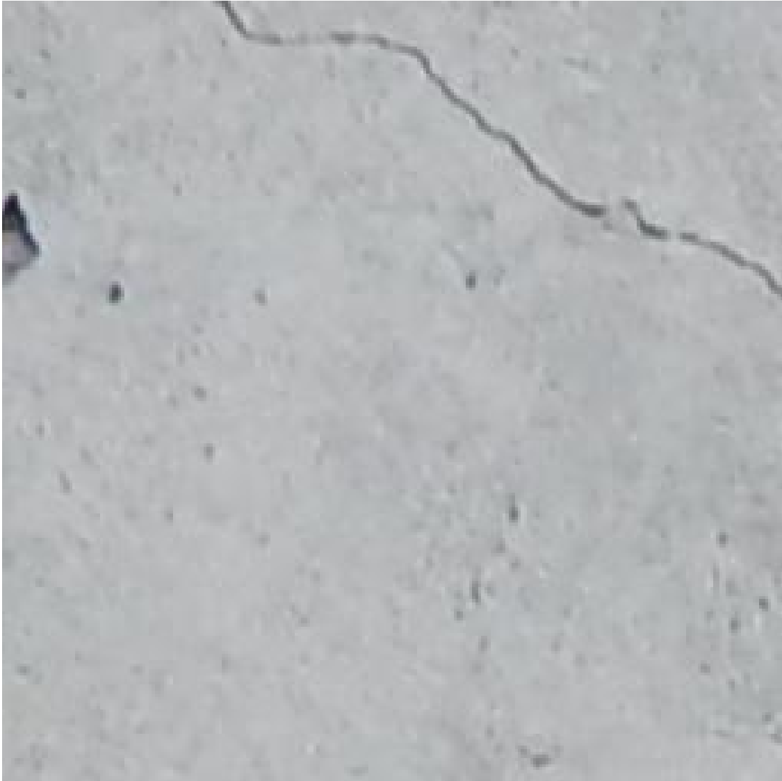
Figure 7.10: Image 7070-24 of a Wall Crack
