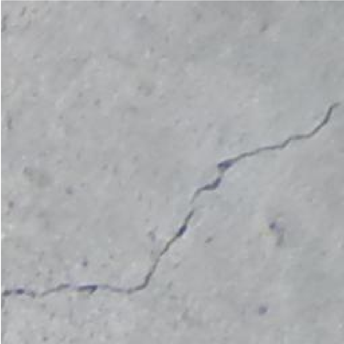
Figure 7.6: Image 7003-18 of a Bridge Deck Crack
