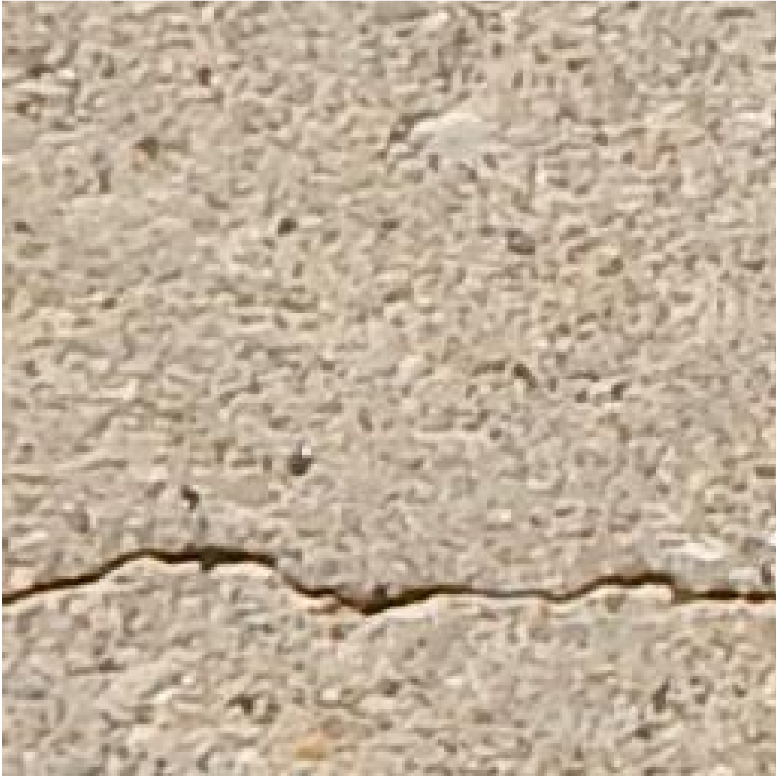
Figure 7.14: Image 004-114 of a Pavement Crack
