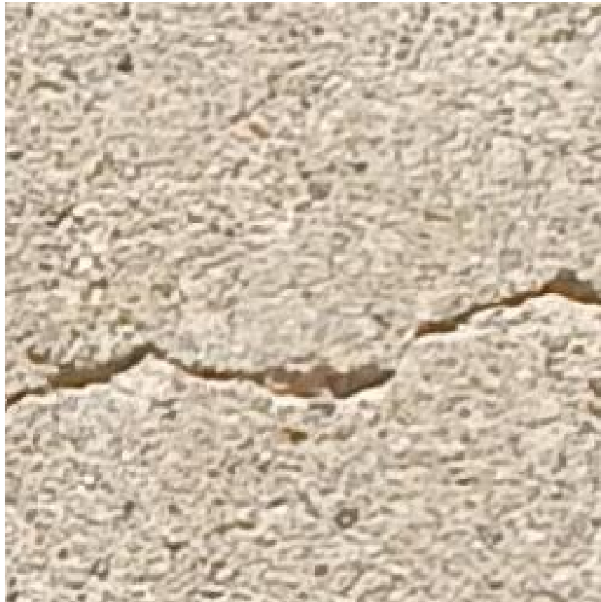
Figure 7.1: Input Image 002-100 of a Pavement Crack
