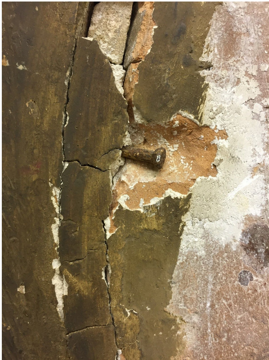
Figure 4: Calligraphic Roundel, Detail of nail between the frame and ceramic roundel, Reverse. Exhibited plaster layer cracking and flaking. Source: Josephine Ren.
