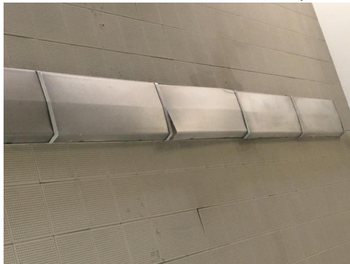
Figure 3. Light fixtures in a room at Western in 2019. One of the light covers is partially loose. By Author.
