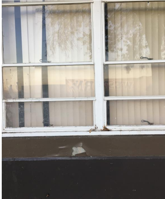
Figure 2. An image of a window of a classroom at Western in 2019. Paint is peeling on the wall, and the window frames are old. By Author.
